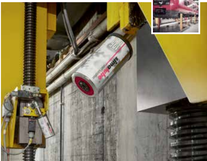
The spindles of a lifting station for railway wagons and locomotives are lubricated with 125 ml simalube over 12 months.
