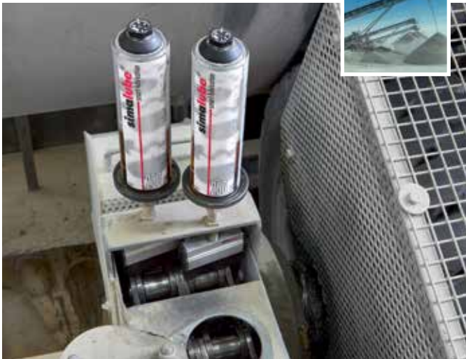
Two 250 ml simalube lubricators with brushes lubricate and clean the chain drive of a drum washing machine.
